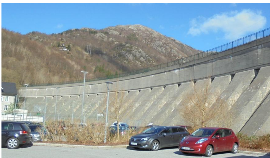
Figur 5 Lamellhodedam, Dam Svartediket (photo: T.Konow).
