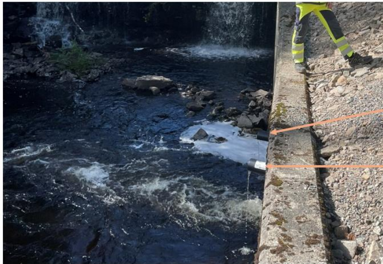
Figure v25. Drains with leakage. One pipe from each side of the dam
