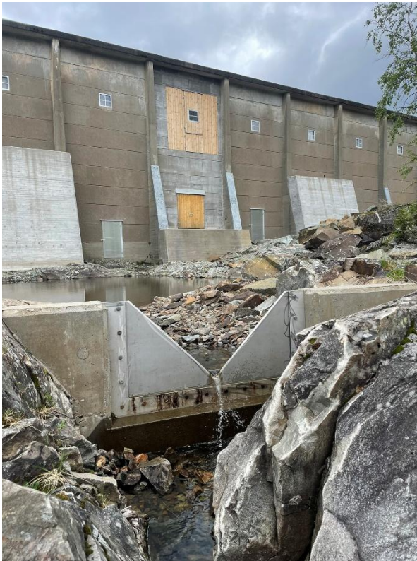
Figure v37. Dam C1 - leakage from the dam with full reservoir, about 0.1 l/s.
