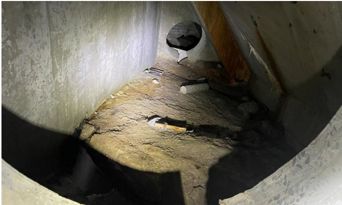
Figure v48. Drainage gallery in front of buttress.
