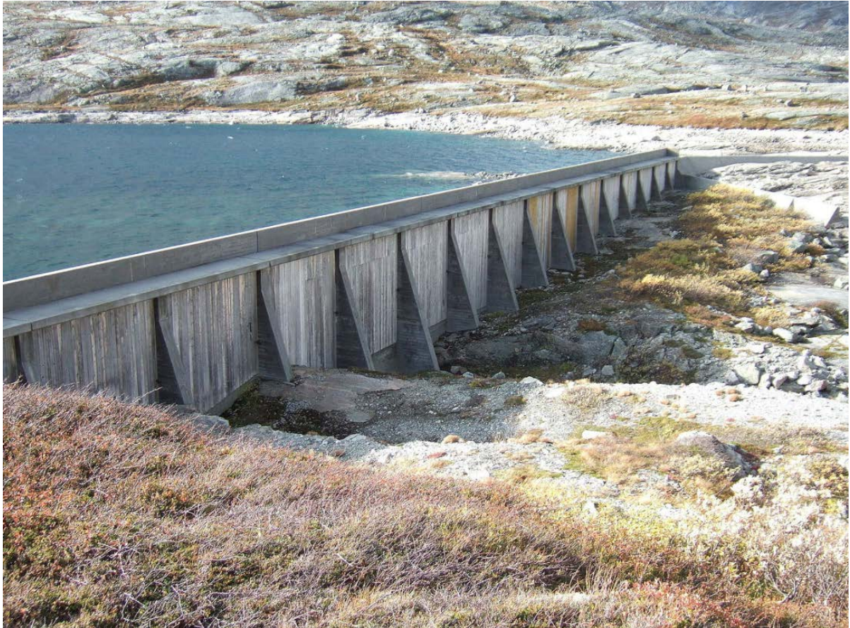
Concrete dam for Fitvannet in Norddal County in Møre og Romsdal (Norway).
