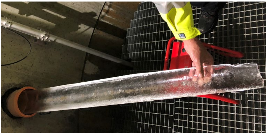
Figure 58: Reduction of leakage volume due to ice blockage.
