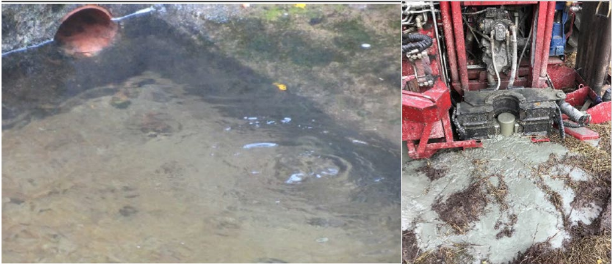
Figure 46: Leakage and occasional discoloured discharge water were observed in the spillway channel (left). High pore pressure is observed in a borehole at the downstream dam toe (right).
