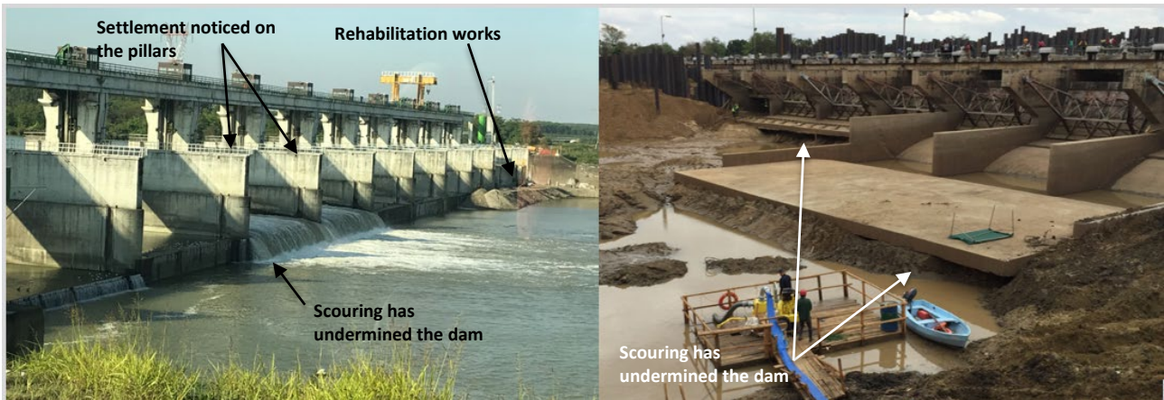
Figure 52: Isola Serfini dam in Italy on the left and Kamuzu Barrage in Malawi on the right.
