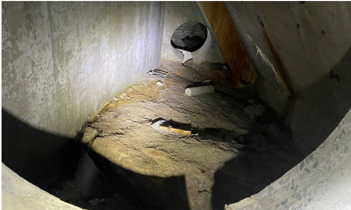
Figure v48. Drainage gallery in front of buttress.
