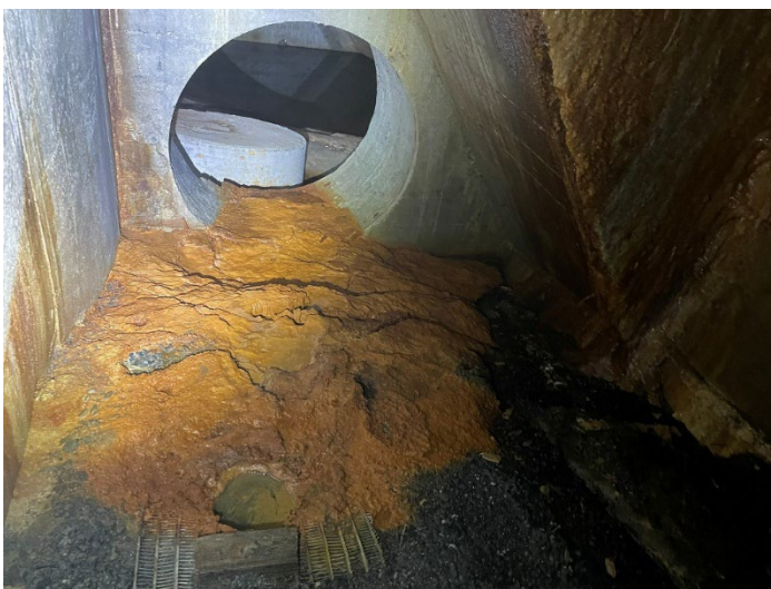
Figure v49. Some of the drains have water seepage with mud-like material from borehole.
